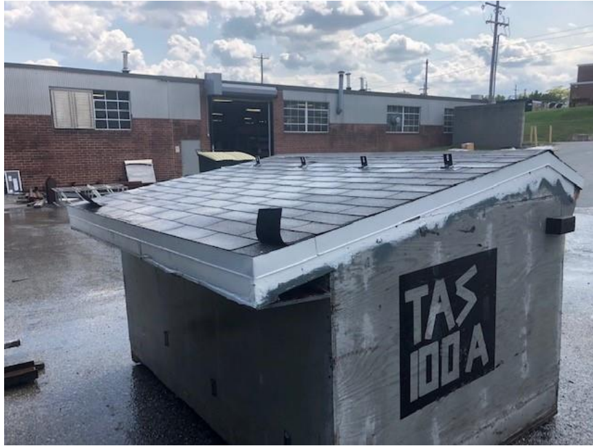
Photo No. 8 70 MPH Top Side After
