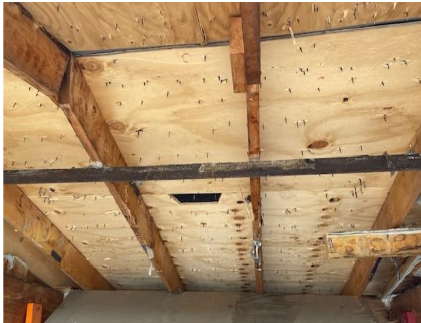
Photo No. 15 Post Test Underside
