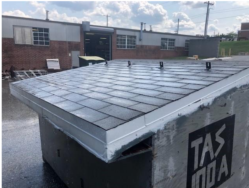
Photo No. 5 35 MPH Top Side After
