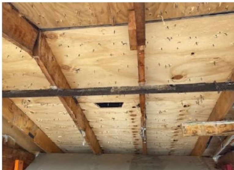
Photo No. 15 Post Test Underside
