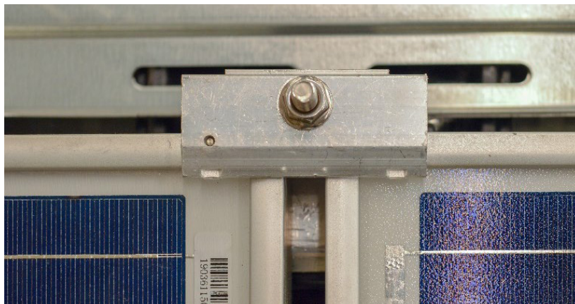
Clamp Securing Two PV Modules
